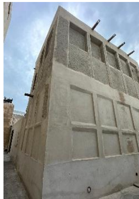
Fig. 10: Well-maintained Source: author
