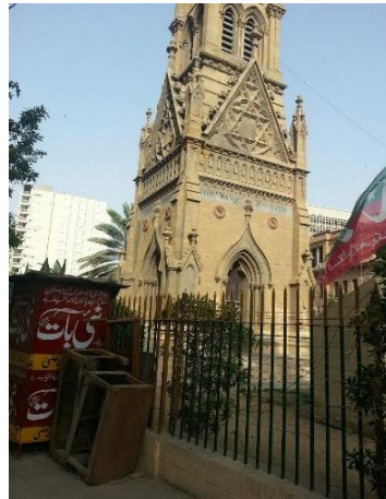
Fig. 12: Lack of Maintenance & Care.
